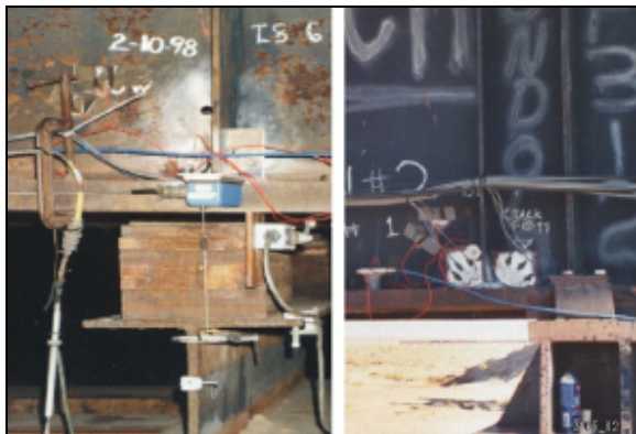
Exhibit 2. Instrumentation at Crack Locations
