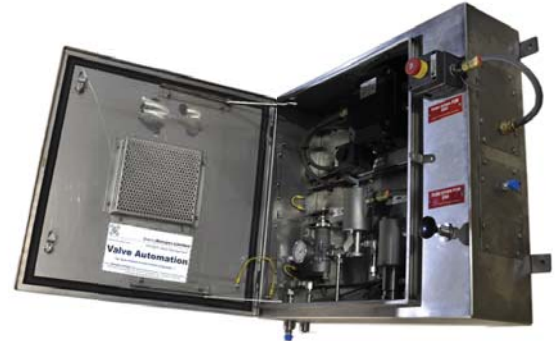
Pneumatic Control Cabinet (ESD / Partial Closure System)
